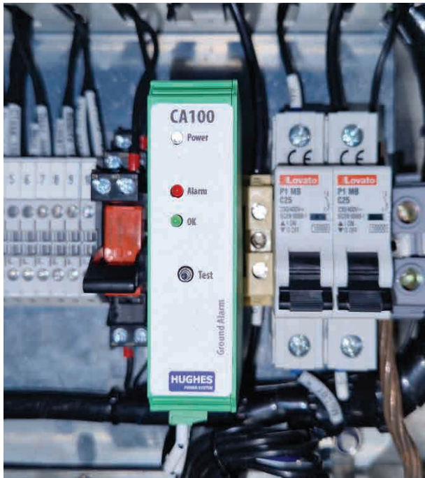
Installation in the motor drive cabinet
